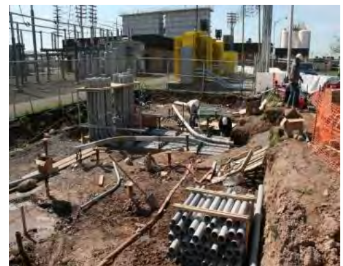
Passaic Valley Sewerage Commission Electrical Substation
