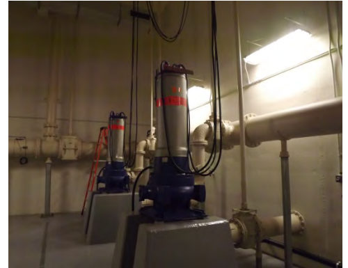
Camden County MUA Pump Station
