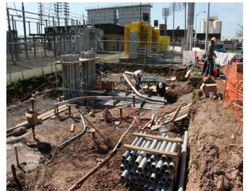
Passaic Valley Sewerage Commission Electrical Substation
