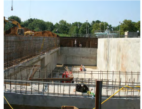
Township of Middletown Sanitary Authority Aeration Digester
