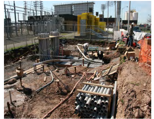
Passaic Valley Sewerage Commission Electrical Substation
