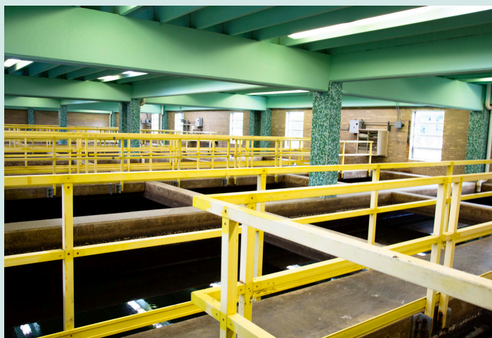
Water treatment in Veolia's Haworth Water Treatment Plant in Haworth, New Jersey.
