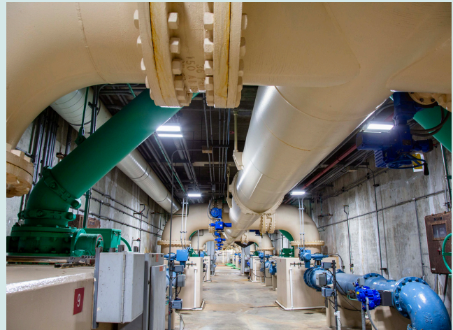
( Top ) Hamden Pump Station operated by the New Jersey Water Supply Authority in Clinton Township, New Jersey; ( Bottom ) Infrastructure located in Veolia's Haworth Water Treatment Plant in Haworth, New Jersey.
