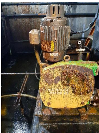
Figure 1: A ferric pump covered in the chemical following a ruptured feed line.
