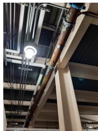
Figure 2: Severely corroded 6-inch utility water line located within the treatment plant.
