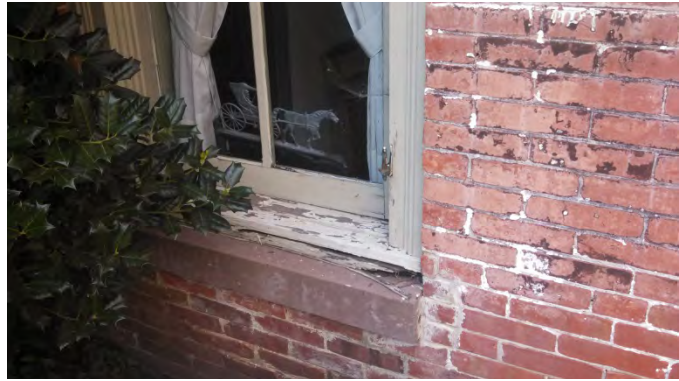
Figure 70: Image showing damage to window trim and brick, at front of Carriage House.
