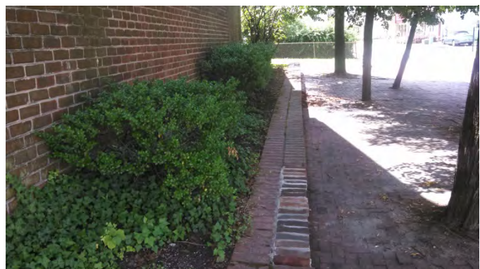
Figure 41: Side planter at the Hoskins House, showing damaged brick and condition at side wall of the house.
