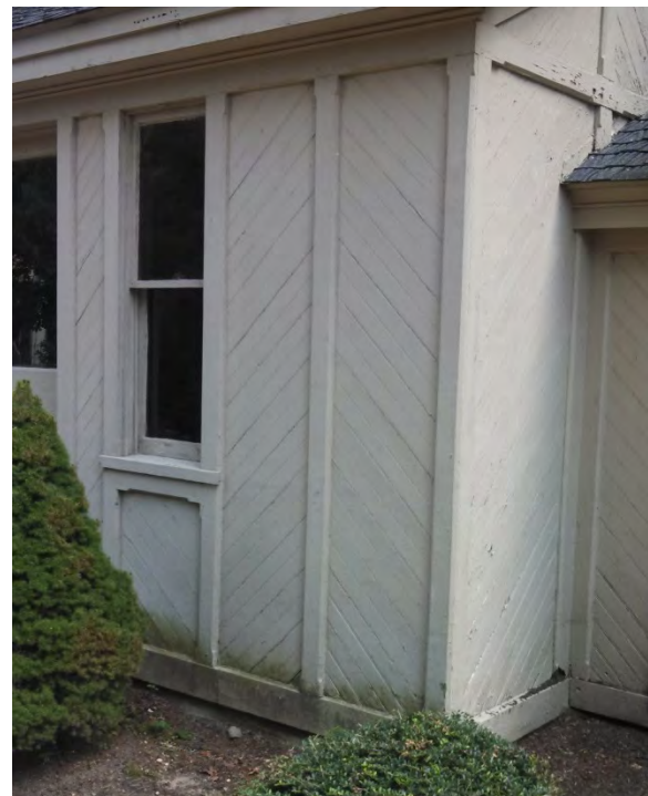
Figure 69: Water damage at base of siding at rear addition.
