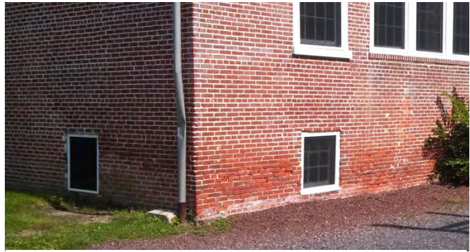
Figure 89: Several of the downspouts have been damaged or are missing.
