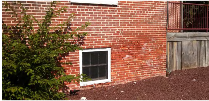
Figure 86: Image of brick damage at the William R. Allen School.
