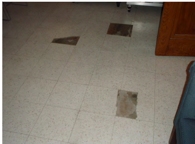
Figure 56: Damaged kitchen floor on the second floor of Lyceum Hall.
