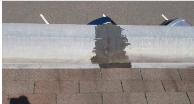
Figure 54: Leaking seam in recessed gutter showing inappropriate repair with asphalt.
