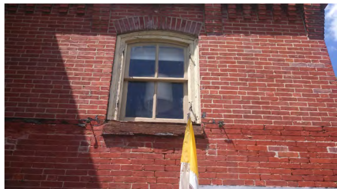
Figure 68: Damaged brick and missing mortar over the main entry of the Carriage House.
