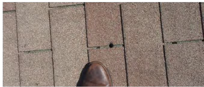
Figure 55: Hole in asphalt shingle roof at Lyceum Hall.
