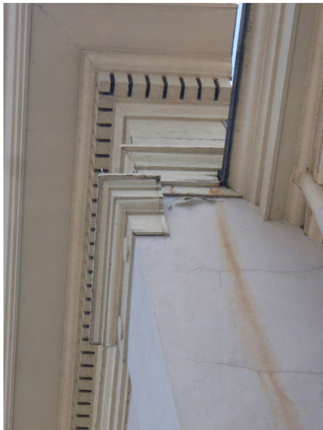
Figure 49: Image of cornice showing typical condition of exterior trim and minor damage/ discoloration of stucco.
