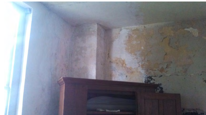
Figure 16: Plaster damage at chimney on the first floor of the Schoolhouse.
