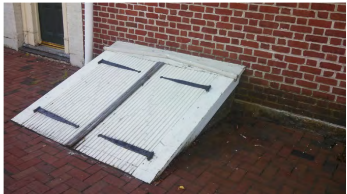
Figure 40: Exterior bulkhead at the Hoskins House requiring repair to prevent water infiltration to basement.
