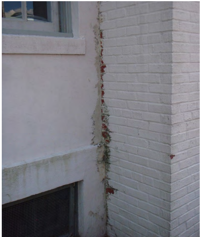
Figure 50: Water damage at brick chimney.
