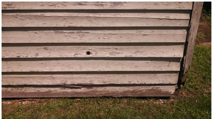
Figure 28: Damaged clapboard at rear addition of Hoskins House.
