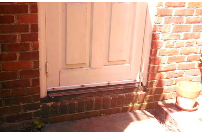
Figure 31: Rear entry showing trim and door damage, as well as step that must be addressed for HC accessibility.
