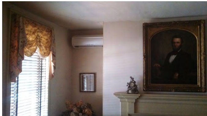
Figure 35: Walls and ceiling in front parlor showing only minor cracks and peeling.
