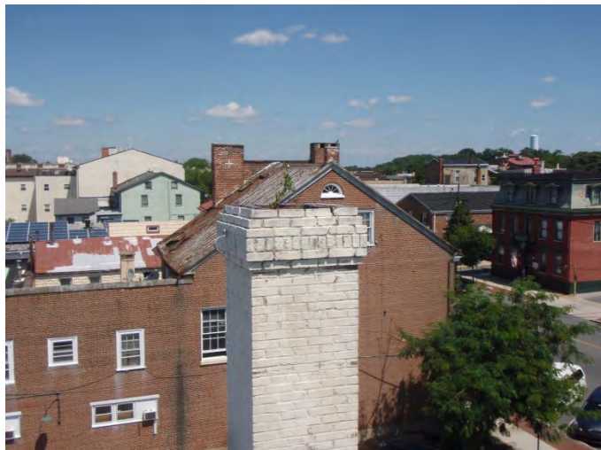
Figure 51: Damage at the top of the chimney at Lyceum Hall.
