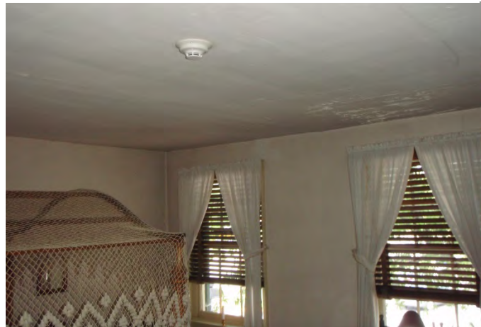
Figure 38: Damaged plaster wall and ceiling in front bedroom on the second floor of the Hoskins House.
