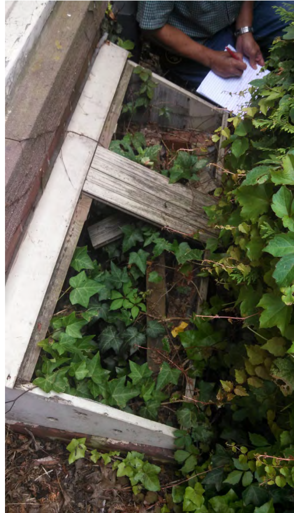
Figure 72: Damaged window well which allows water infiltration into basement.
