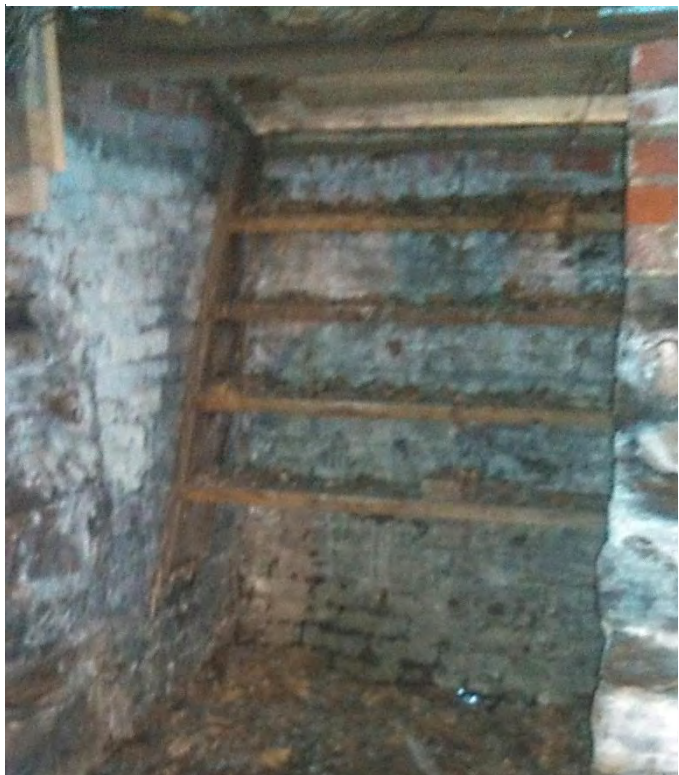
Figure 18: Damage to steps from the bulkhead due to water leaking.
