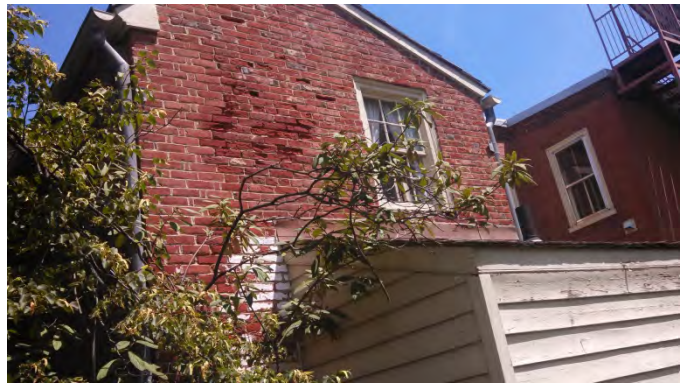
Figure 27: Rear of Hoskins House showing damaged brick.
