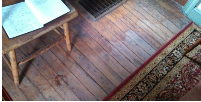
Figure 73: Water damage on flooring near main entry to the Carriage House.
