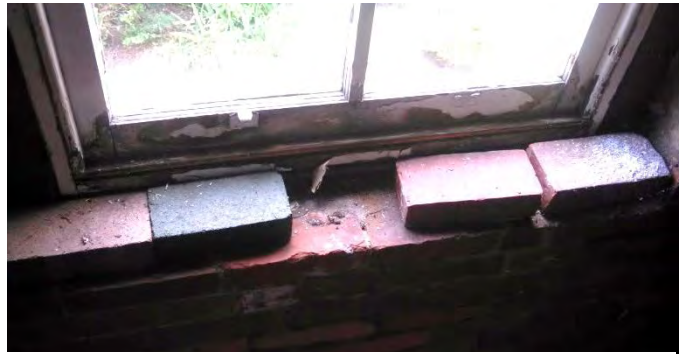
Figure 76: Loose brick at windows on second floor. Note window sash requiring repair and repainting.
