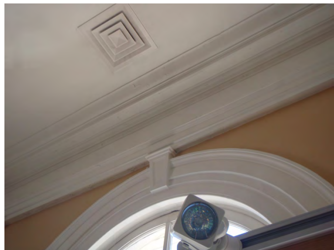
Figure 58: Minor peeling paint at decorative cornice in 2nd floor front room.
