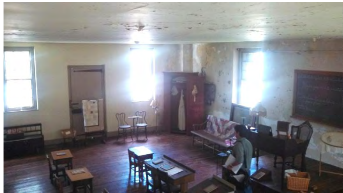
Figure 14: Interior view of the Schoolhouse showing condition of plaster and good condition of floors.
