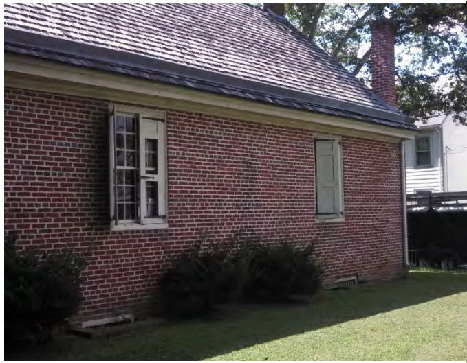
Figure 13: Damage to shutters at Quaker Schoolhouse.
