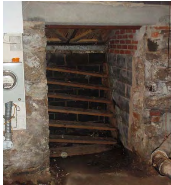
Figure 39: Image of steps to bulkhead, damaged by water infiltration.
