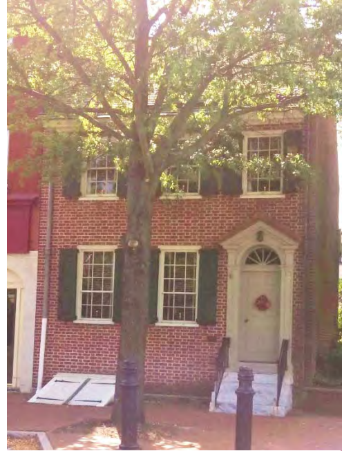
Figure 32: Front elevation showing damaged shutters.
