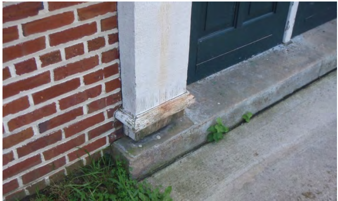
Figure 87: Damage to wood trim at front door.
