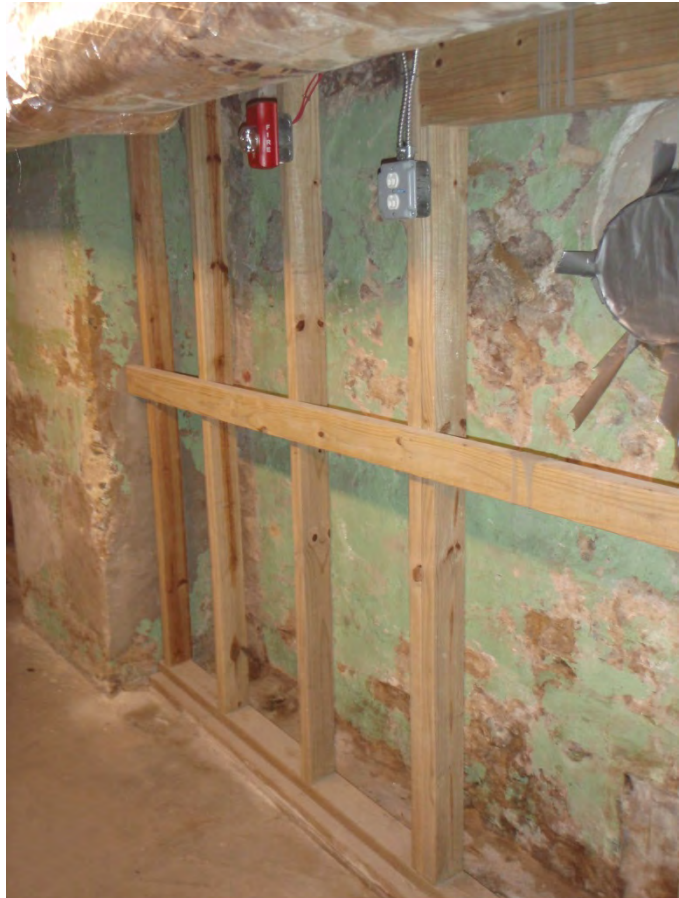
Figure 57: Minor damage to basement walls. Water leaking should be resolved when the chimney is capped.
