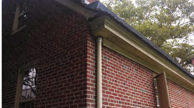
Figure 12: Photo showing downspout replaced with PVC pipe and some damage to the fascia/ cornice at the Quaker Schoolhouse.
