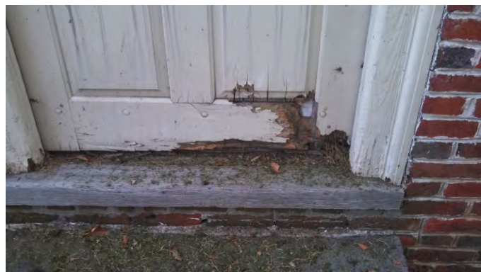
Figure 11: Damaged door at entrance on left side of the Quaker Schoolhouse.
