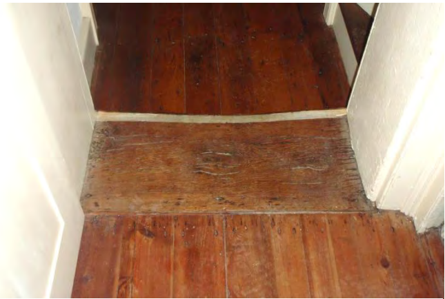
Figure 34: Typical condition of the floors in the Hoskins House.
