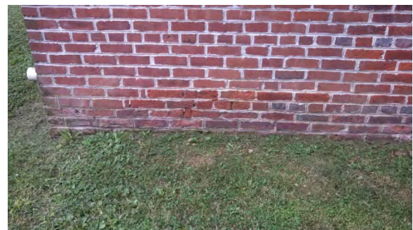
Figure 9: Damaged bricks at the Quaker Schoolhouse.
