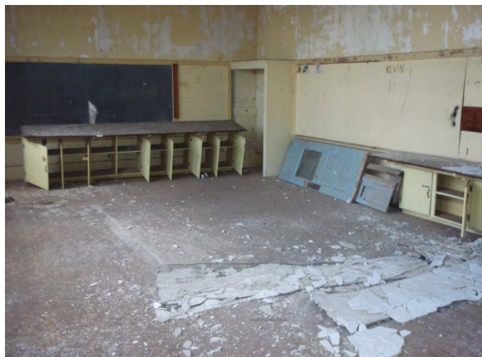
Figure 93: Classroom with collapsed ceiling.
