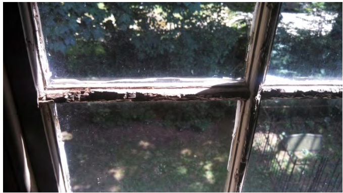
Figure17: Damage to interior of wood windows on the second floor of the Schoolhouse.
