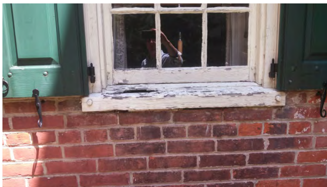
Figure 30: Typical sill at the Hoskins House in poor condition.
