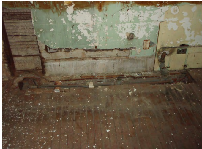
Figure 91: Floor and plaster conditions at the William R. Allen School.
