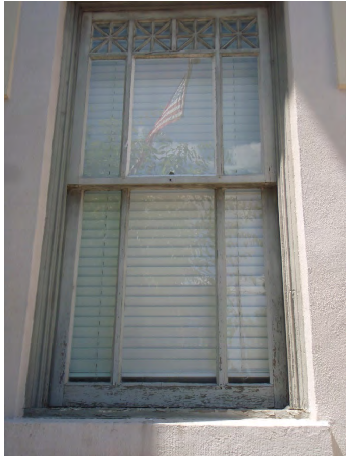
Figure 52: Front window at Lyceum Hall showing typical condition (repainting and re-glazing required).
