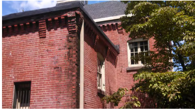
Figure 67: Brick damage and staining at the front left corner of the Carriage House.
