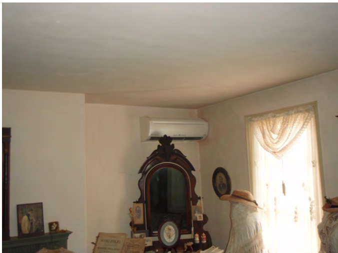
Figure 36: Somewhat more plaster damage in the second bedroom on the second floor of the Hoskins House.
