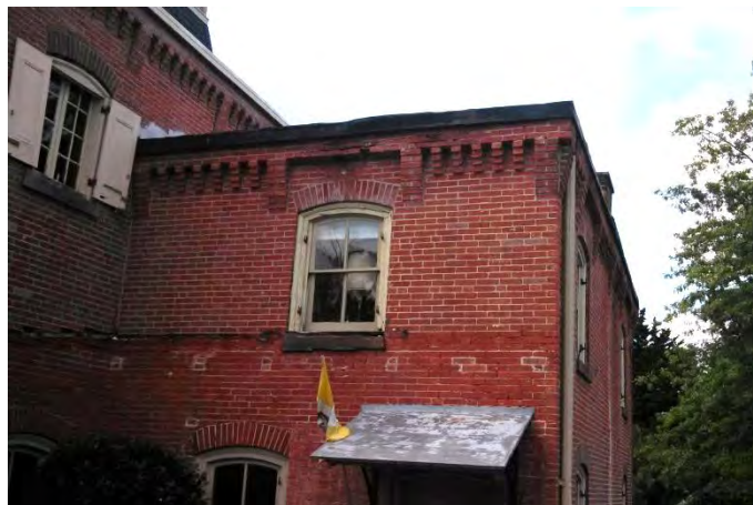
Figure 71: Low-slope roof portions of the Carriage House are particularly poorly detailed, allowing water to drip over the edges and damage brick.
