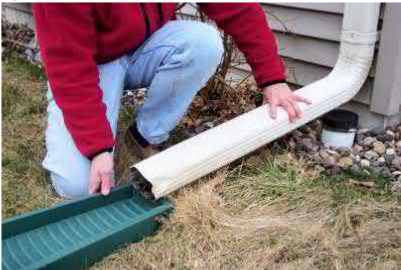
Figure 4-5 - Photo of Disconnected Downspout
