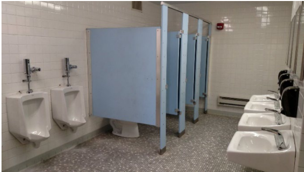
Ocean City Intermediate School restroom with newly installed high efficiency WaterSense certified toilets, urinals, and faucet aerators.
