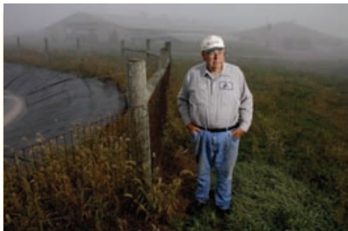
In 1996 New York dairy farmer Bob Aman installed a manure storage and anaerobic digester system to reduce odors on his 500-cow property. In 2004 the generator produced nearly 400,000 kilowatt-hours of electricity, more than what the farm used that year.
