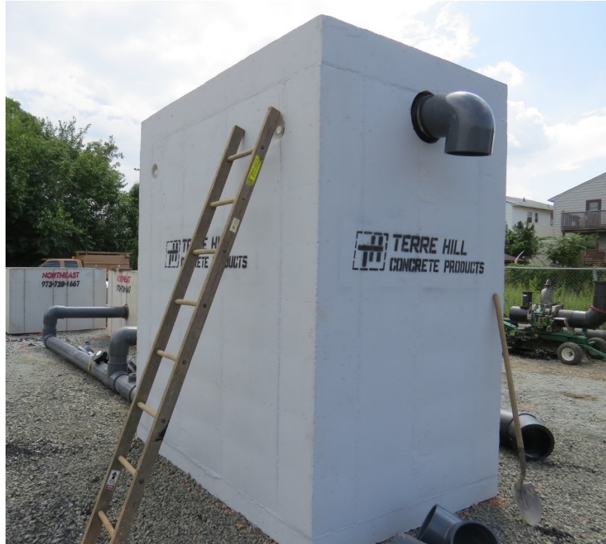
Figure 4.2 Terre Kleen TK-09 unit delivered to site
