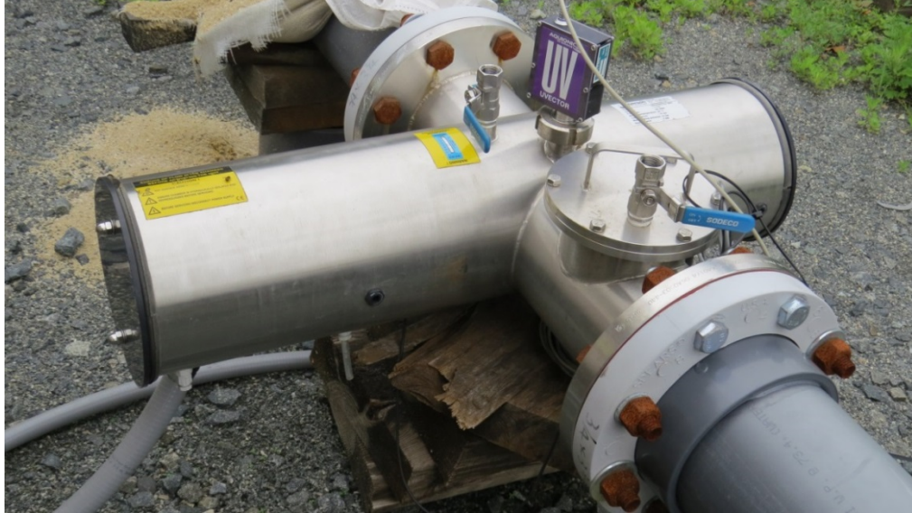
Figure 4.9 Aquionics UV 250+W Unit used in project
