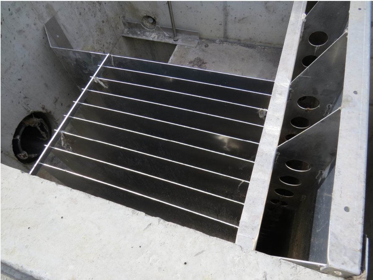
Figure 4.3 Terre Kleen TK-09 unit interior
