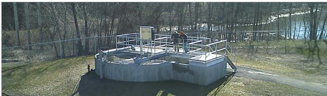
The Storm King® system treats flow prior to discharge into the Saco River (pictured in the background).
