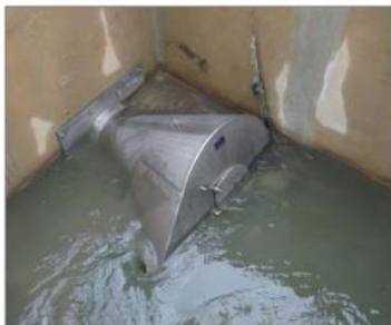
Two Hydro-Brake® Vortex Valve flow controls are used at the Saco CSO Treatment Facility
