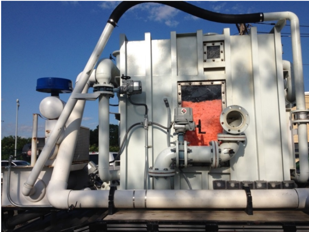
Figure 4.7 Westech WWETCO FlexFilter unit delivered to site
