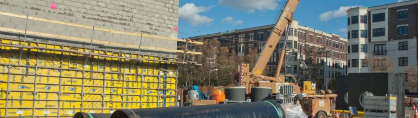
Bergen County Utilities Authority Joint Meeting Pump Station
